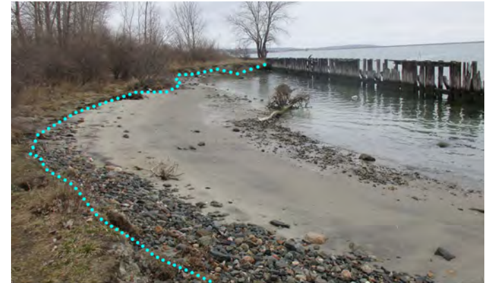
Inland erosion issues - South Harbor
