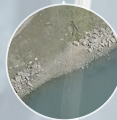
BREAK in wall
