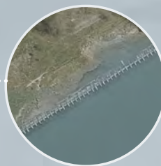
EROSION behind bulkhead
