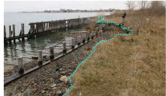
Inland erosion issues - Central Harbor
