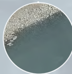
UNSTABLE rubble walls
