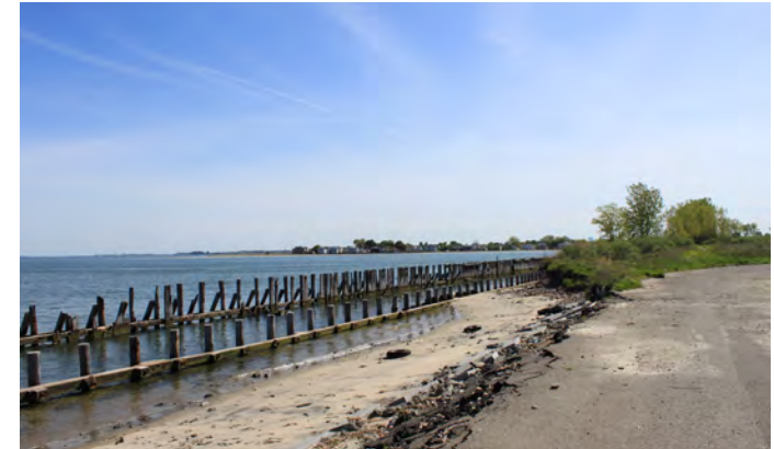
Existing sea edge deteriorating behind Walmart
