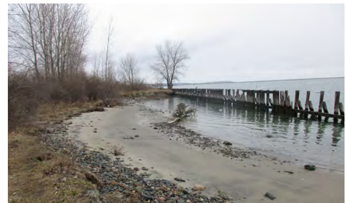
Erosion landward of deteriorated timber bulkhead wall
